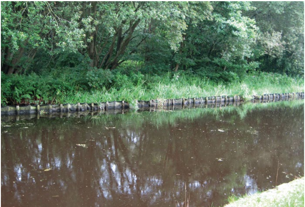
A marginal reserve for Luronium natans constructed on the Huddersfield Broad Canal c.2002 using geotextile curtain and wooden posts. Seen here in August 2019, it has been colonised by Glyceria maxima (Reed Sweet-grass). Ray Goulder
