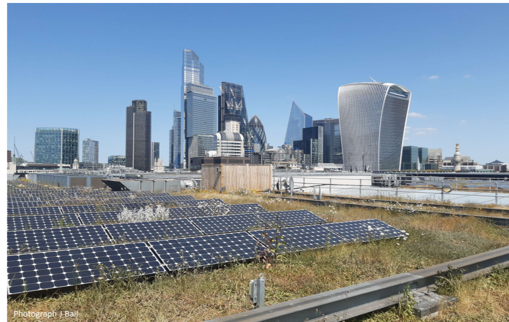
Figure 1. Eleventh Floor Sedum Conversion Roof in the City of London – Nomura International Plc.
